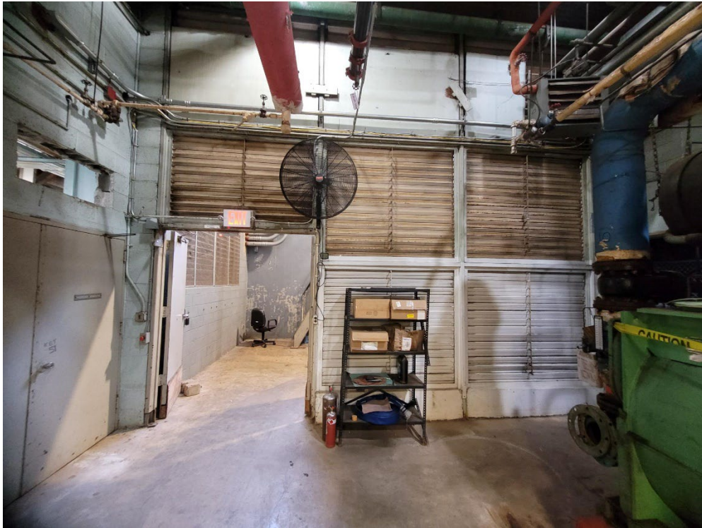
Louvers that may require removal to facilitate new chiller installation.
