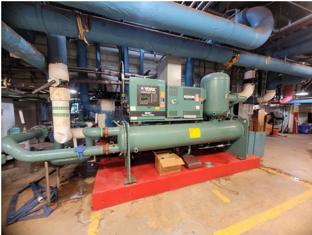
Chiller #1 to be evaluated and possibly replaced.
