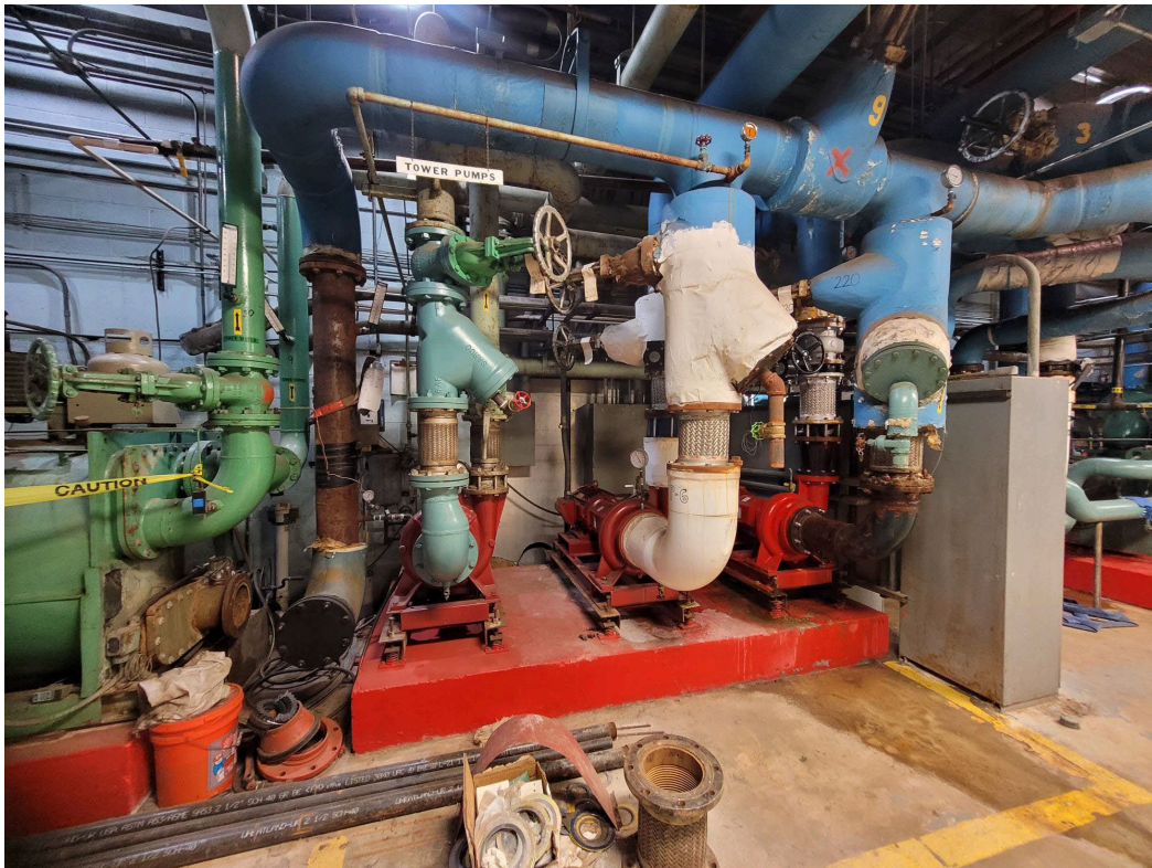
Pumps for chiller #2.
