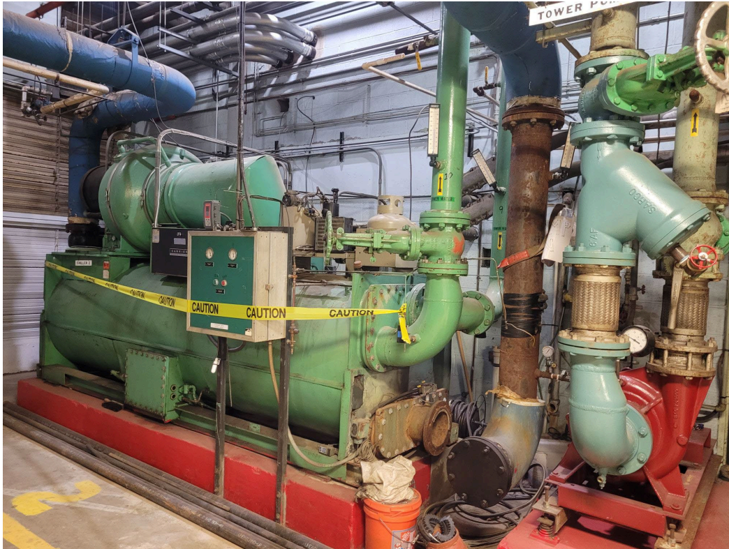
Chiller #2 to be replaced. Note louver doors that may need to be removed.
